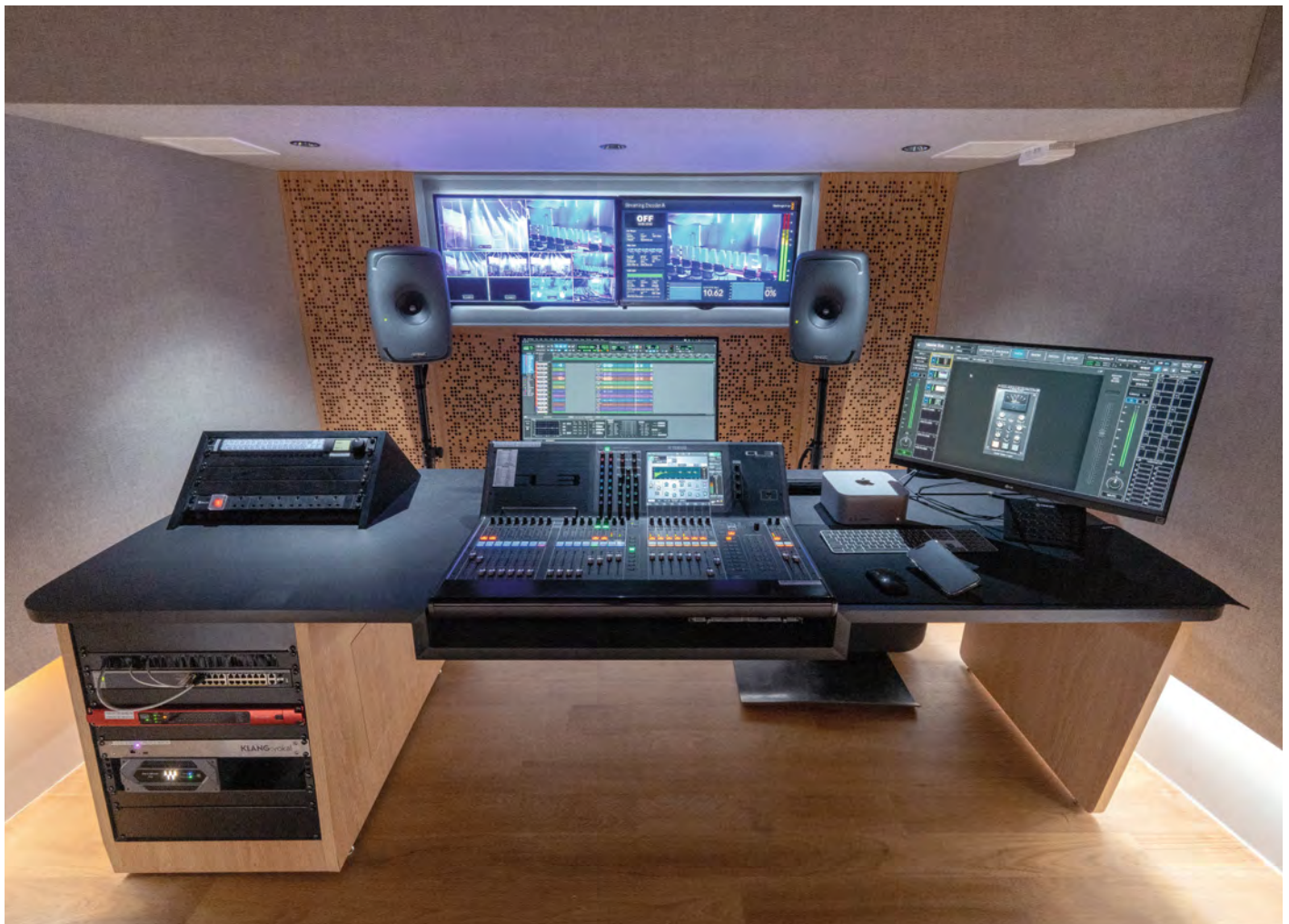
Broadcast streaming is enabled from a Waves Soundgrid Server and a Yamaha CL3 console
