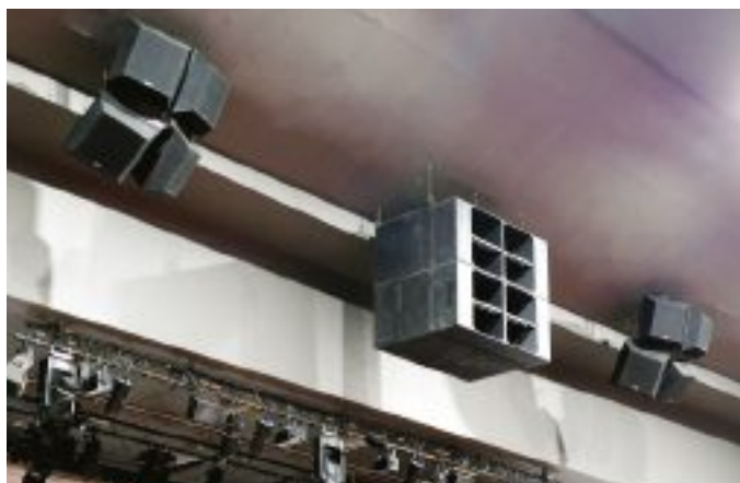
The EAW FOH loudspeaker system combines Quad 12-inch QX models with SB1002 subwoofers
