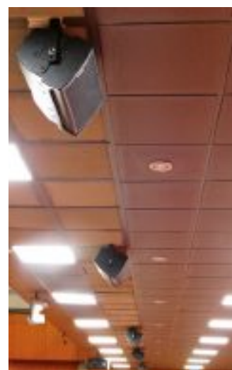
EAW MK2396i speakers provide first tier upper balcony-fill coverage
