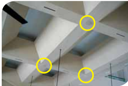
25 units of C8 Community ceiling loudspeakers were installed at the Main Prayer Hall
