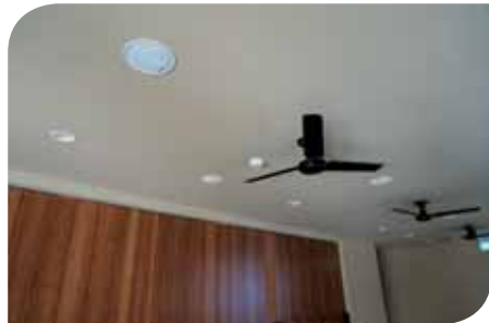
EAW CIS300 4" ceiling speakers installed across the mosque.
